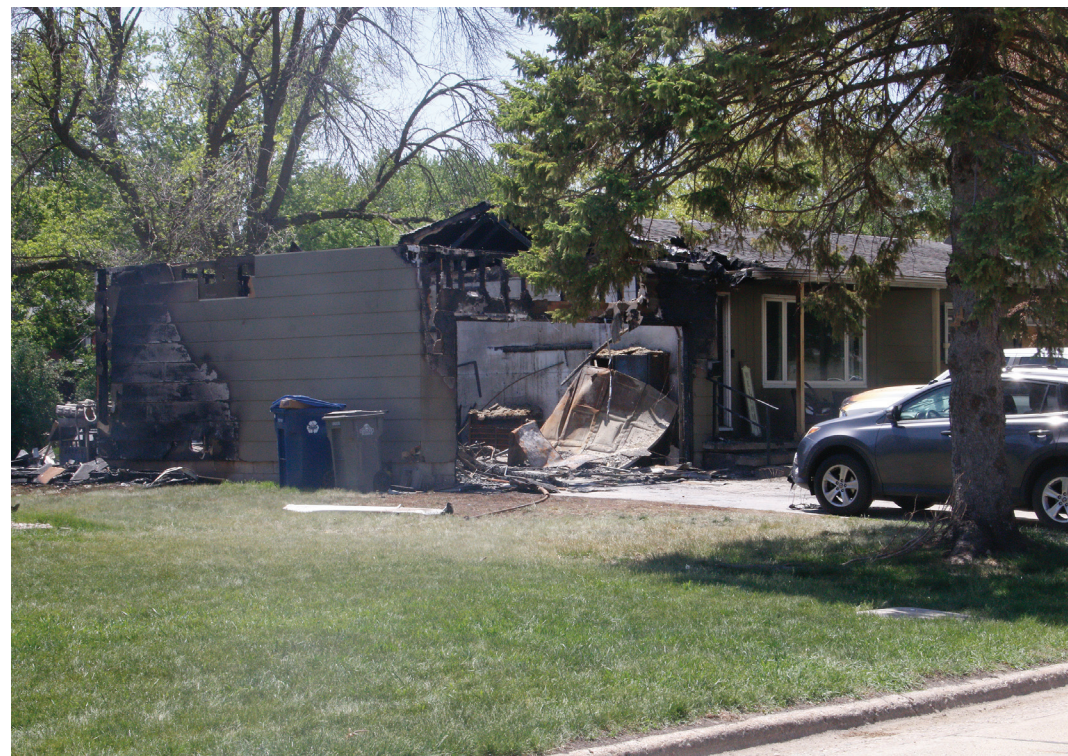
Garage and attic area of a home sustained significant damage in an evening fire on Wednesday, May 13, on East 19th Street. No injuries were reported, according to the Spencer Fire Department. (Photo by Carol Grace Riner)
