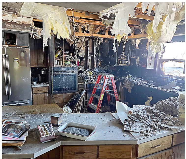
The aftermath of the fire at the David and Janice Willert home east of Rockford.
