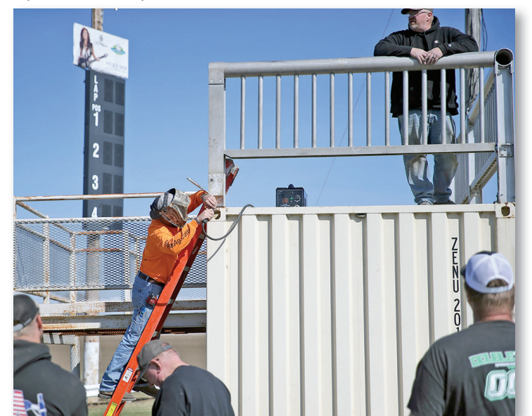
Duston Anderson welds a piece of railing to the upgraded Judges/Announcer's Stand Saturday morning at the Cedar County Raceway in Tipton. The stand is one of several planned upgrades to the Raceway located in the Cedar County Fairgrounds throughout the season. As a result, the March 28 Spring Fling has been called off, but racing will begin this season on April 16.
